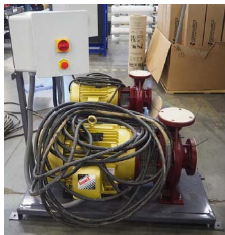
Figure 25: Example Media Filter Supply Pump
